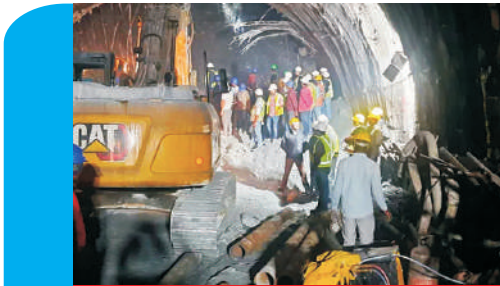
Silkyara-Barkot Tunnel Collapse
